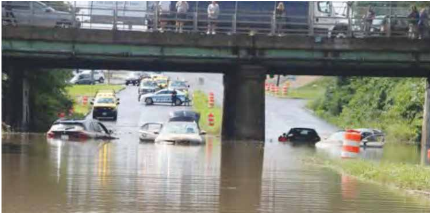
Candidate resiliency project under development: Flood relief on Route 20 / Route 122 interchange, Worcester
