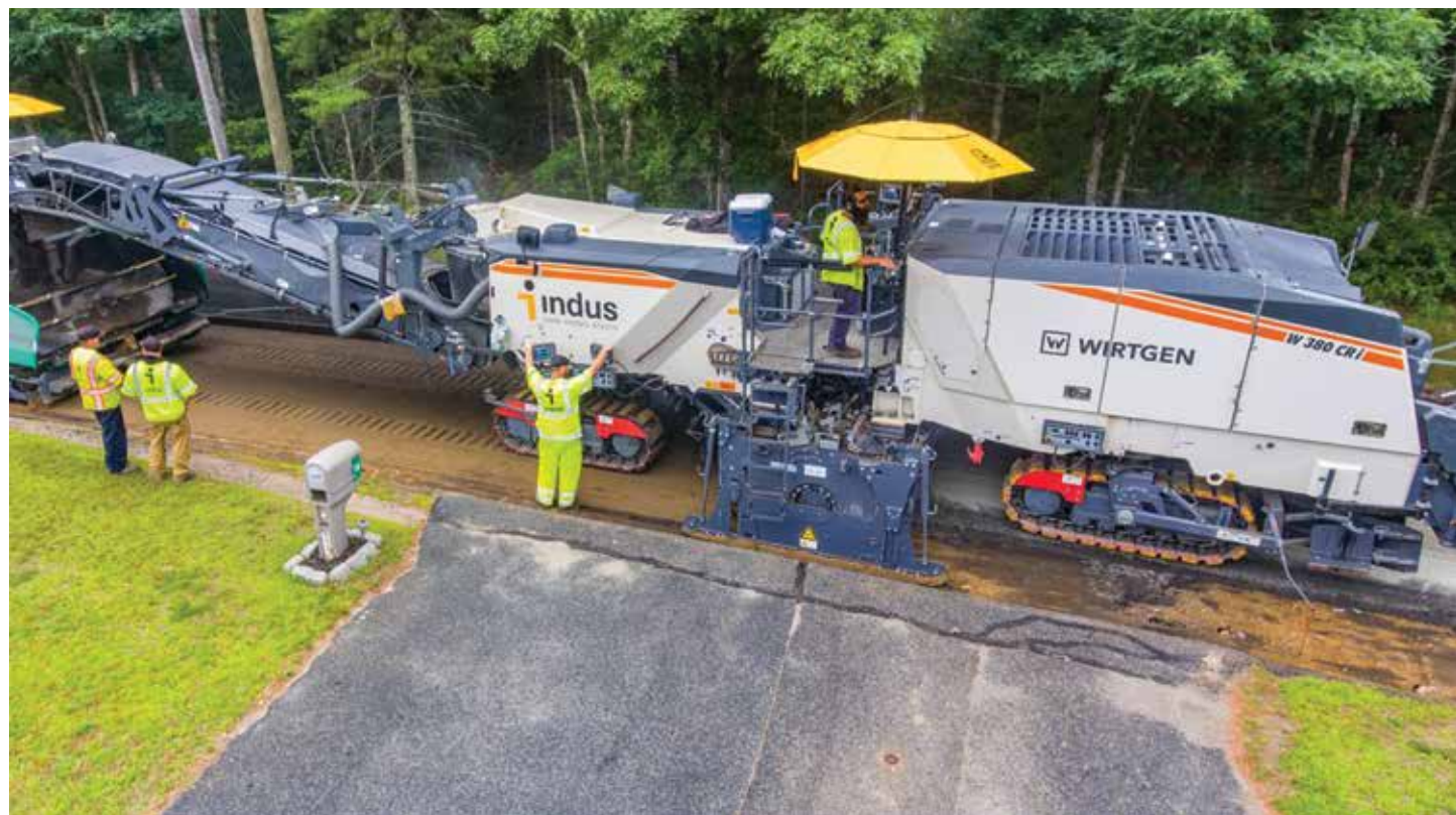
For additional information regarding Paver-placed Stabilized Full Depth Reclamation, please reach out to Art Baker art.baker@indusinc.com For more information on PPSFDR indusinc.com/roads/paver-placed-stabilized-full-depth-reclamation/
