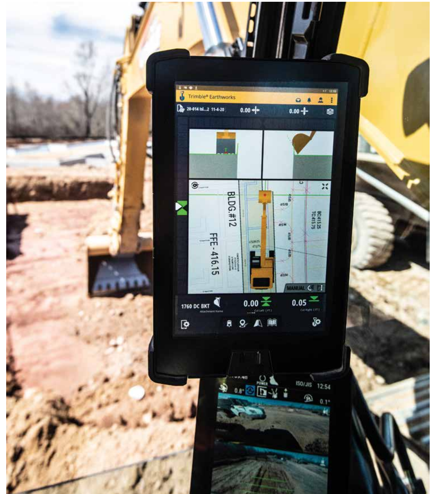
A foundation design model uploaded to the Trimble Earthworks software in a CAT excavator.
